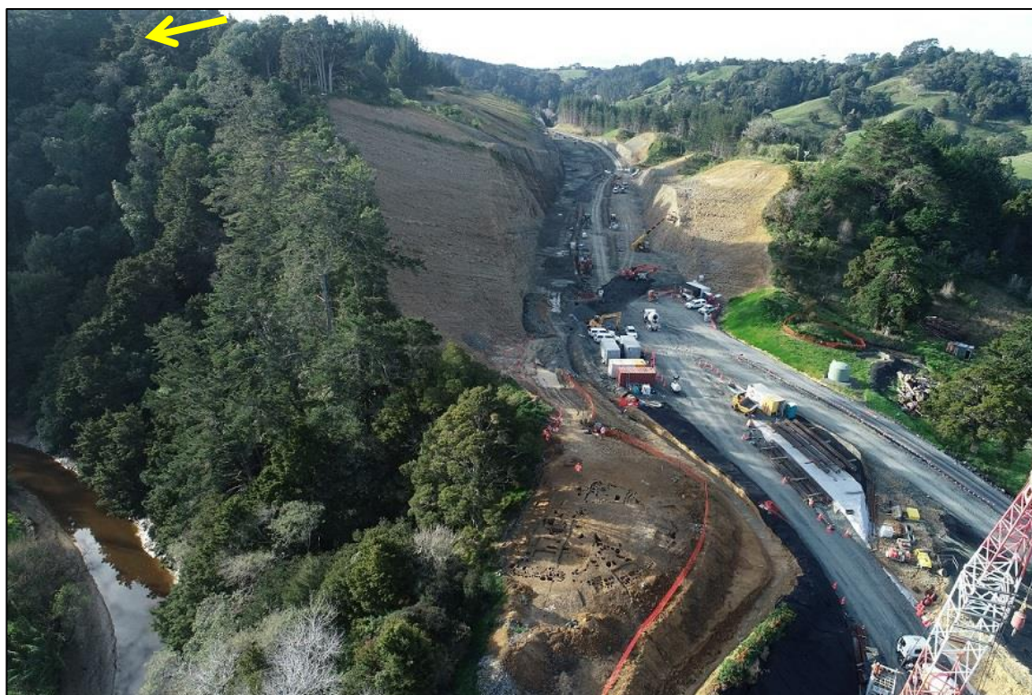
Figure 4.74 Oblique drone-captured aerial image showing the R10/1417 upper terrace site and enclosure (centre bottom) following excavation, with the location of a possible kāinga at the top of the scarped embankment (arrowed)
