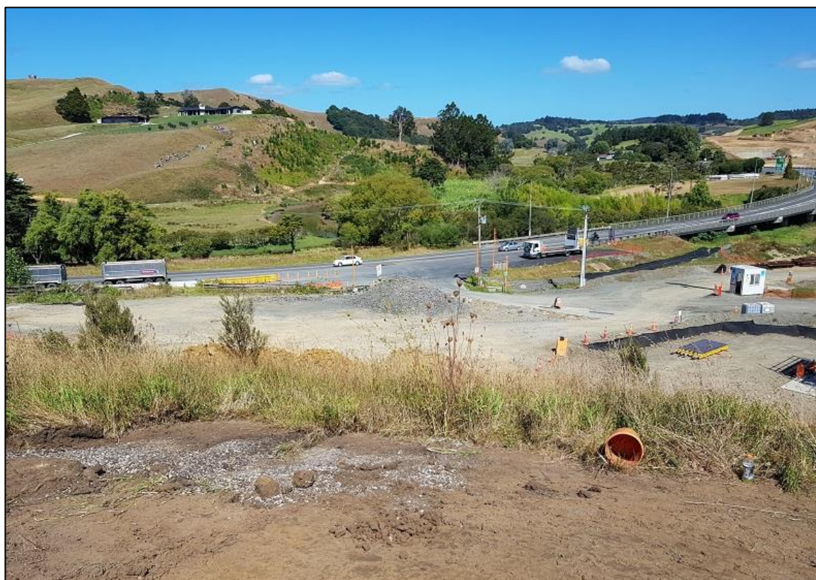
Figure 4.105 Shell midden deposit (3048) on the lower terrace of site R10/1417 seen during topsoil stripping in February 2019; facing southeast
