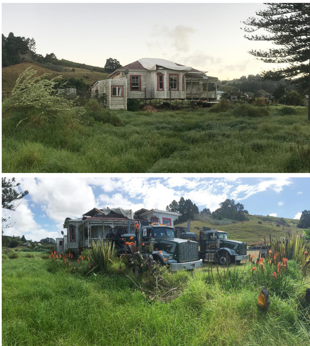
Figure 3.99. Images of Schollum House being lifted – top, and placed onto flatbed trucks for relocation (bottom)
