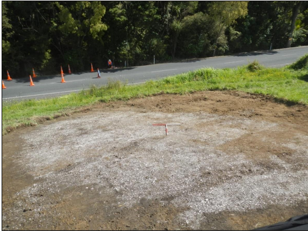
Figure 3.35 North facing view across site R10/1498 at 3 Puhoi Road, prior to excavation. Scale: 2 x 1m
