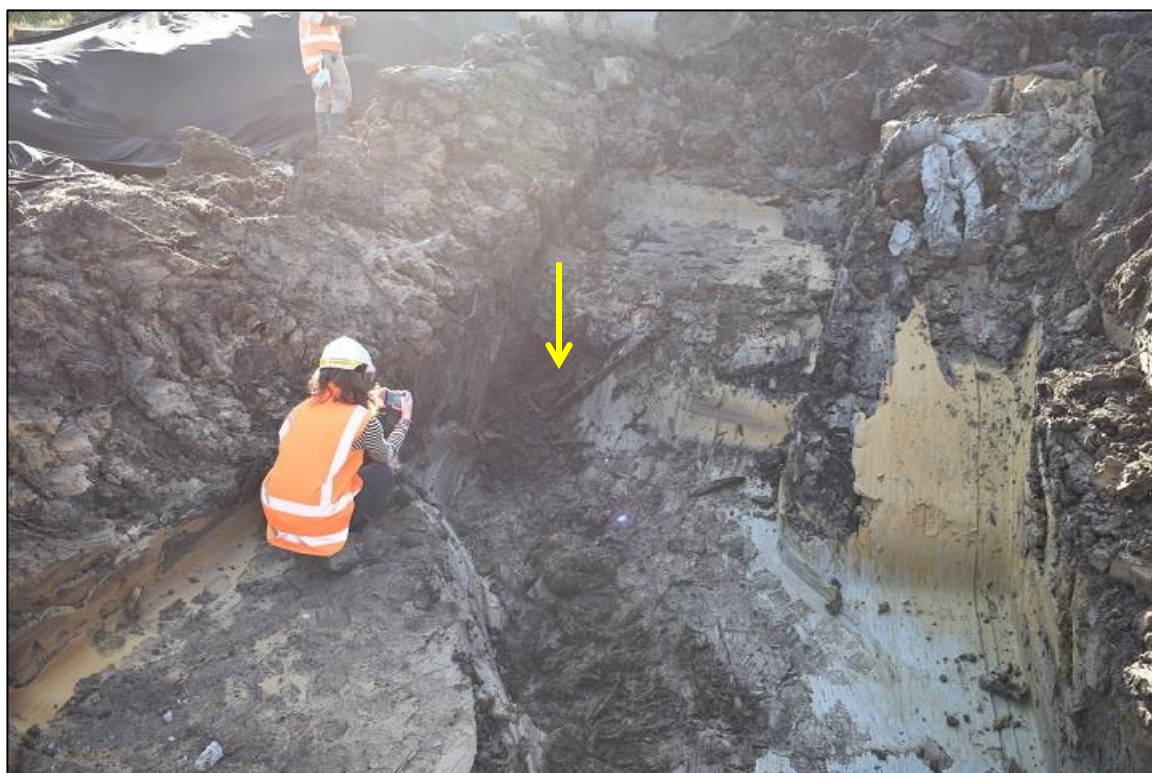
Figure 3.103 The flood deposit as it was exposed by the mechanical excavator during drainage works situated to the immediate west of Carran Road, approximately 2.5km to the west of Warkworth
